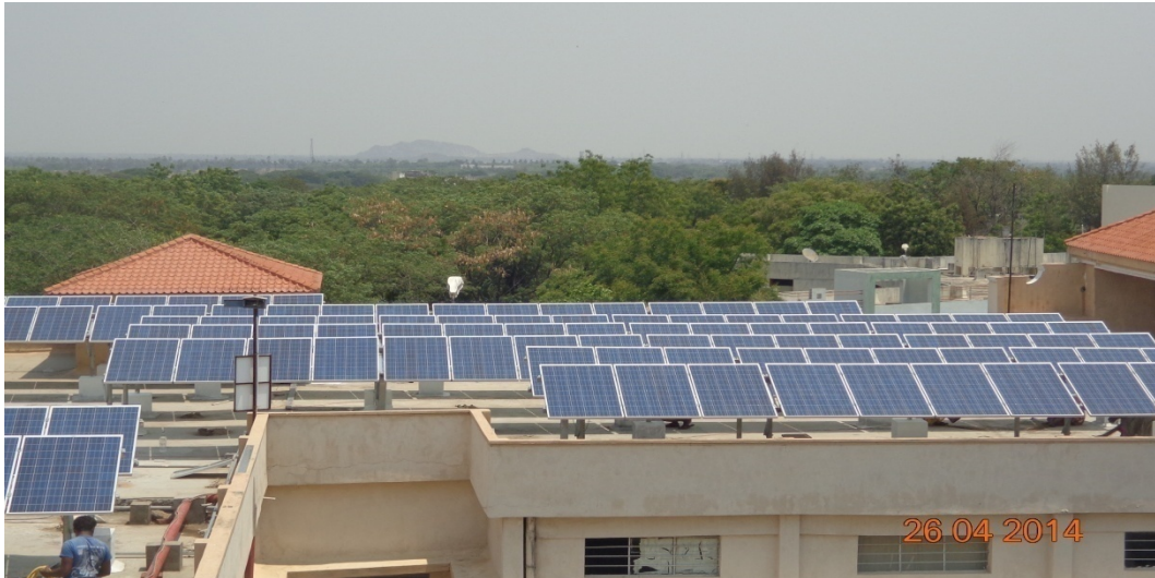
Fig- Roof Top Solar Energy Generation system
